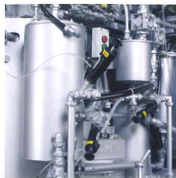
Avoids creation of odor: the water separator system
